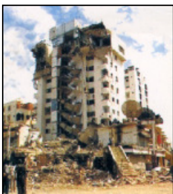
Fig. 3.3a: Destruction caused by an Earthquake in Gujarat
