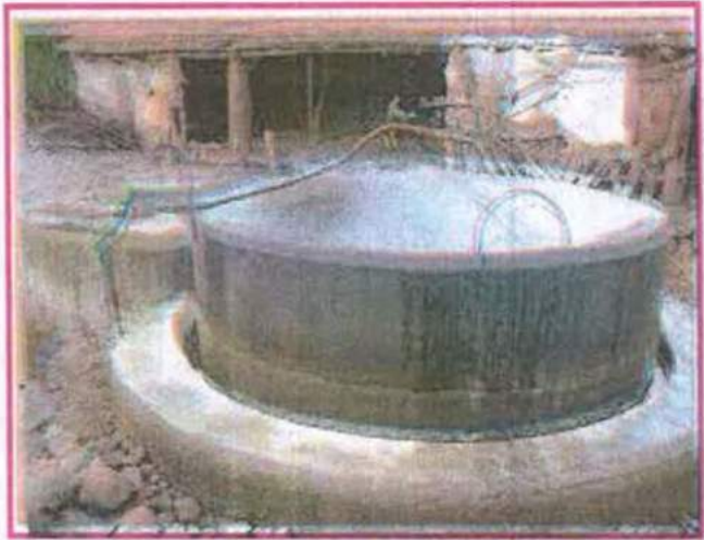
Fig. 1(D). 14: Biogas Plant
